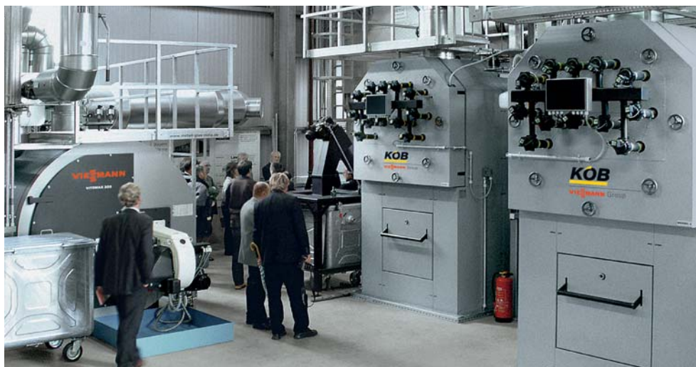
Biomasse-Heizwerk Markt Schwaben Biomass heating plant in Markt Schwaben, Germany
